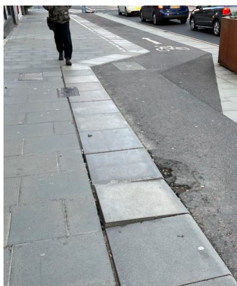
Very narrow pavement in area of high footfall; post hoc widened for cyclists following international press coverage (is remaining space for the planter really necessary?); rocking slab is a hazard for pedestrians; potholes near lip increase risks for cyclists
