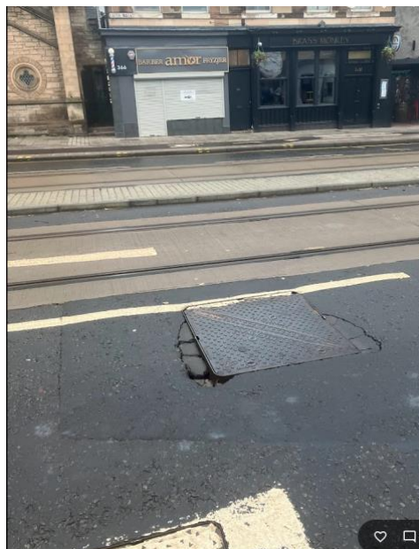
Photo taken NOV 23, barely six months after "start of revenue service": worn out lines, previous repair attempts, against A-listed building in the background; not the high-quality environment we were promised (damage still there and getting worse)
